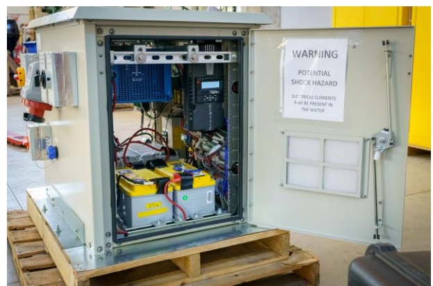
Fig. 3. A picture of the final power electronics enclosure that was deployed in North Carolina, USA, in 2022 (image credit: Andrew Simms, NREL)
