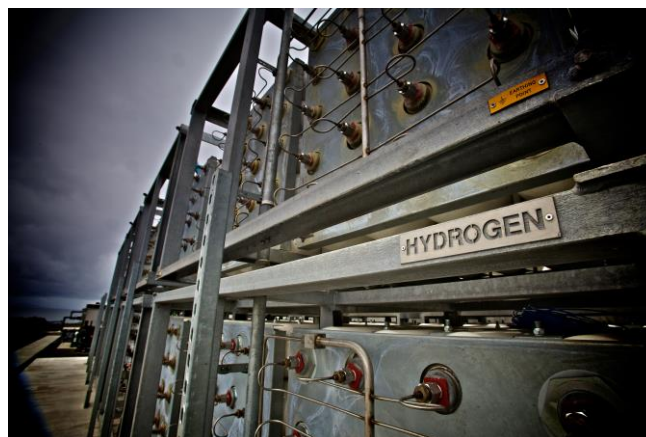
Fig. 3. EMEC Hydrogen Production Plant on Eday [4]
